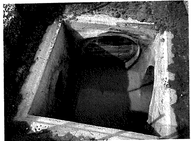
Example - Storm installed.
