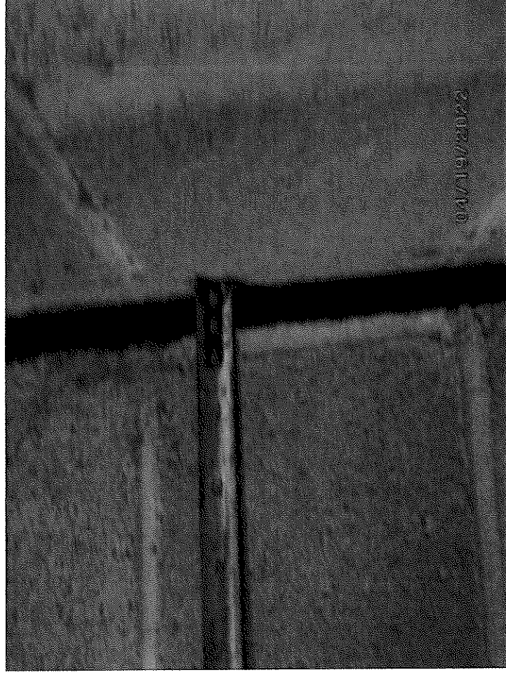
Wall bowing approx. \frac{3}{4} " away from column
